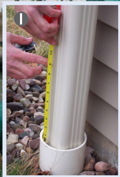
1 Measure 23cm from top of sewer standpipe. Measure higher if using rain barrel.
